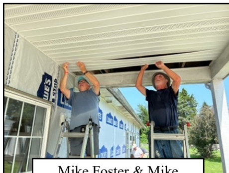
Mike Foster & Mike Schmook installing soffit on entry porch of the building
